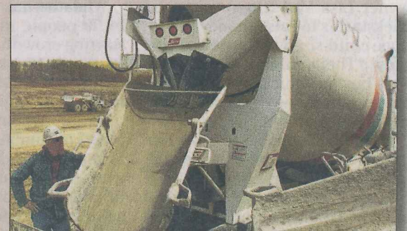
PRESQUE ISLE DOWNS & CASINO: Avery Schou, of E.E. Austin, delivers concrete grout into a pump at the Summit Township site in 2006.
