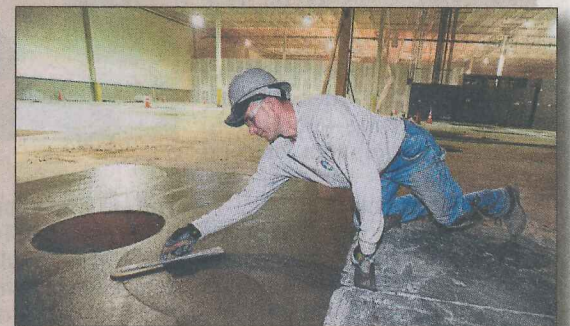
LORD CORP: Eric Andree, a concrete finisher with E.E. Austin, works at the company's new Summit Township facility in 2013.
