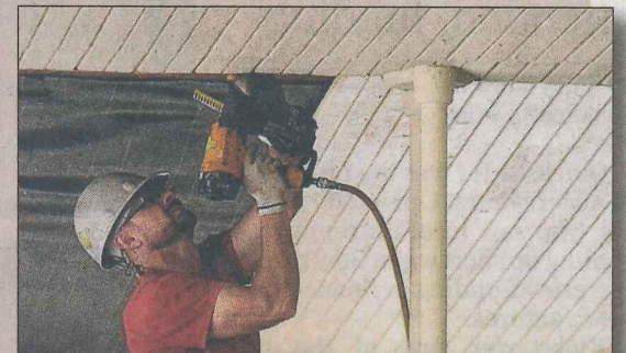
CHAUTAUQUA INSTITUTION: Jason Muscarella, of E.E. Austin & Son, installs boards on the amphitheater ceiling in June.
