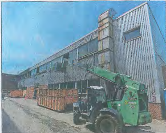
The Erie School Board on Monday awarded a $435,000 bid to Erie-based E.E. Austin & Son to demolish a burned-out section of Erie High School and install a structural steel shell and temporary walls.
